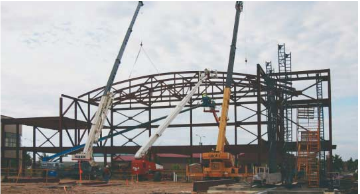
Bow-string trusses are skylined at the North Dakota State University Health and Wellness addition in Fargo, N.D.
