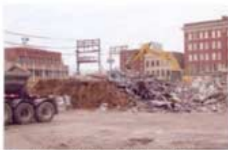
Demolition of the Lark Theatre/Cinema Grill in downtown Fargo makes room for the new Cityscapes Plaza.
